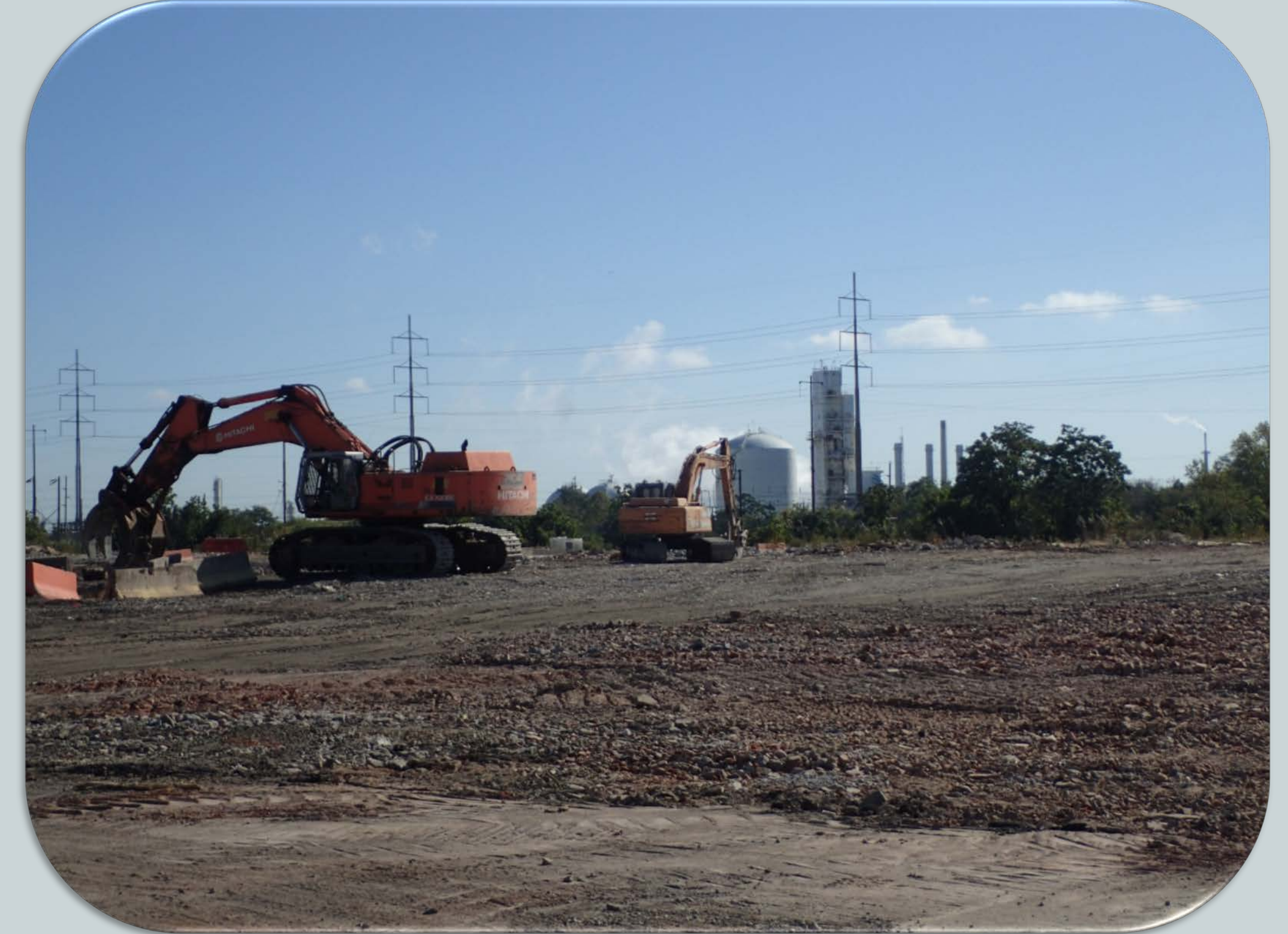
Excavators prepare the Citi Steel site near Claymont for redevelopment. Photo by Susan Love, DNREC.
