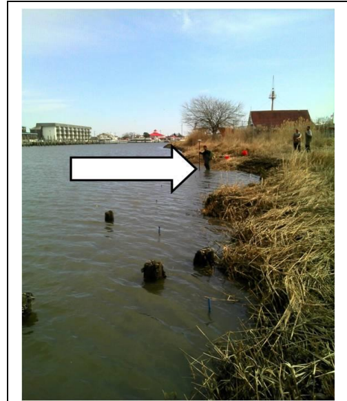
Figure 2 Eroding marsh edge in the Lewes Marsh site treatment area. The large cusp behind the white arrow is located directly across the canal from a marina boat ramp.
