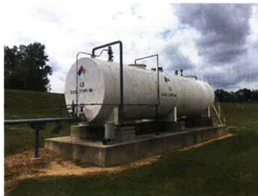
12,000 gallon tank at New Jersey facility
