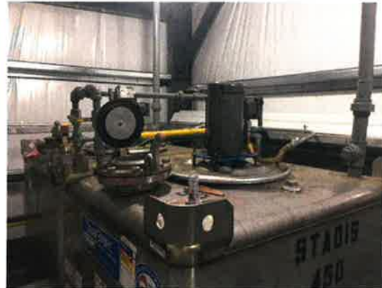
250-gallon metal tote – NJ facility
