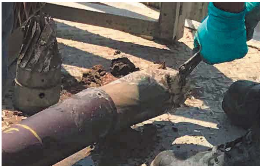
Photo 4. Removal of Plastic Sleeve and Sample Material from Pole. Vibracoring Cone on Left.
