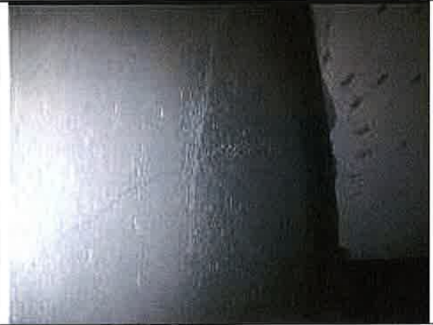
Stage 1 HPT Shroud Crack Servieable
