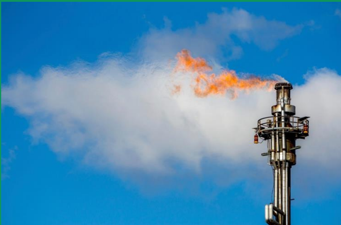
This is a representation of a flare during use. Image used with permission courtesy of CleanAir.com/tag/flares/
