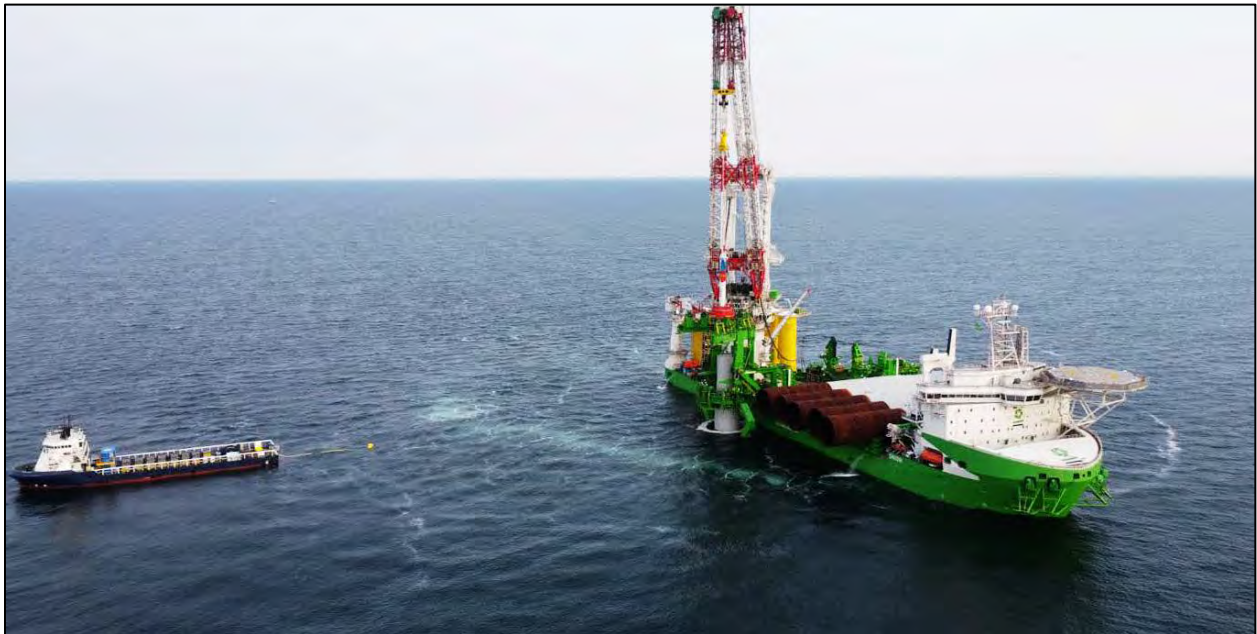
Figure 1. The Orion, drone view, in Vineyard Wind lease area. Photo by DEME [1], shows Orion (right) at stationary position with hammer on starboard side, monopile sections in laydown amidships. Bubble curtain support vessel at left.
