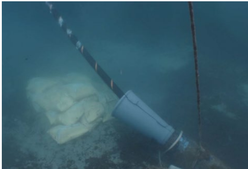
Figure 2.1-8. Underwater View of Near Shore Cable Pull into HDD Duct (Source: Nexans.com)
