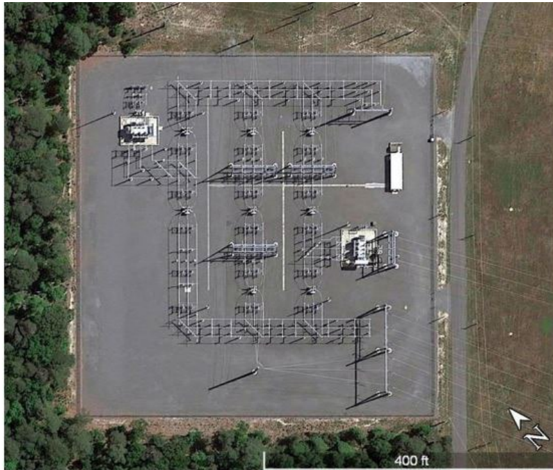
Figure 2.1-6. Indian River Substation
