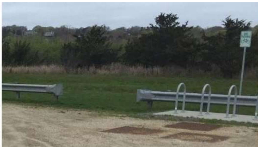
Figure 3.1-15. Typical Vault within Parking Lot Post Construction
