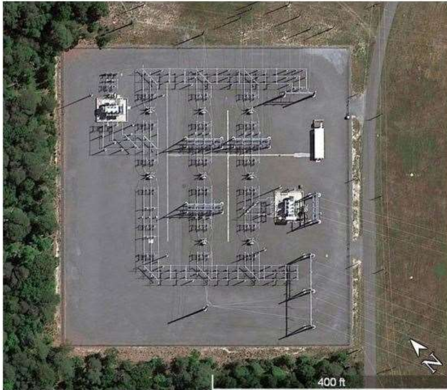
Figure 3.1-18. Indian River Substation
