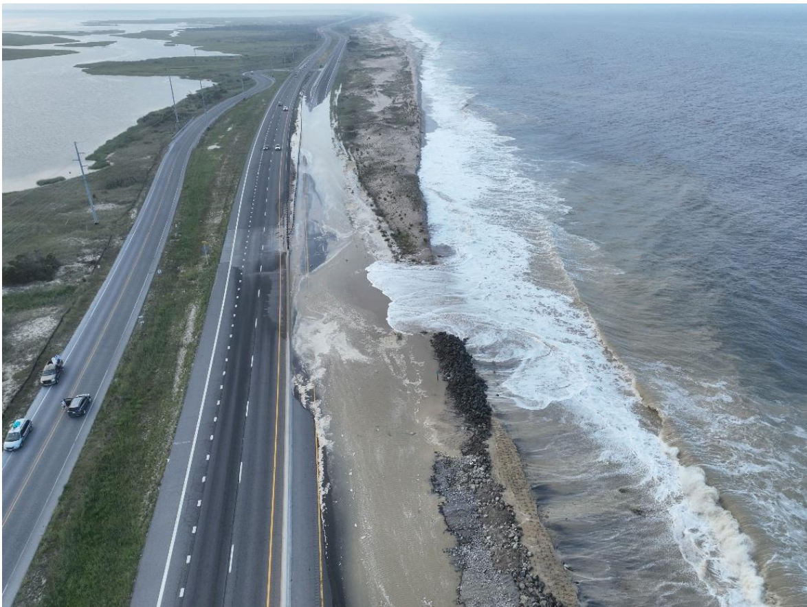
Figure 2. August 17, 2024. Aerial view of the dune breach at Delaware Seashore State Park (looking north). The SR-1 northbound lane is closed to vehicles and completely covered in ocean water, sand, and debris.
