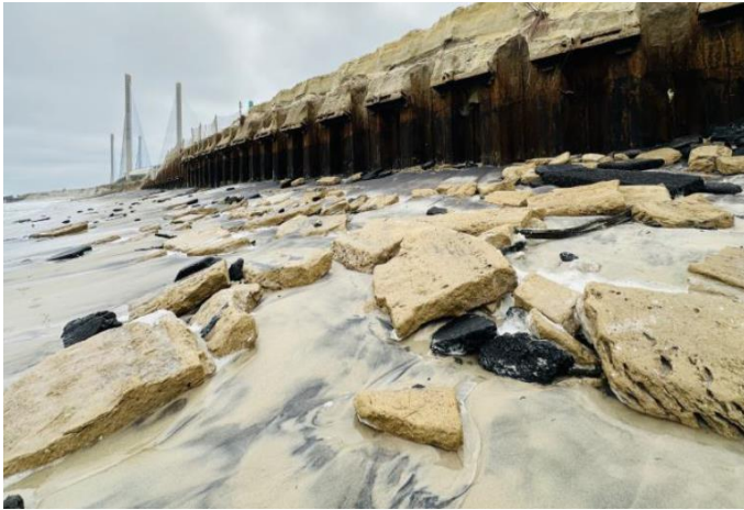
Figure 4. April 2024. View (looking south) of hazardous debris exposed on North Beach due to erosion
