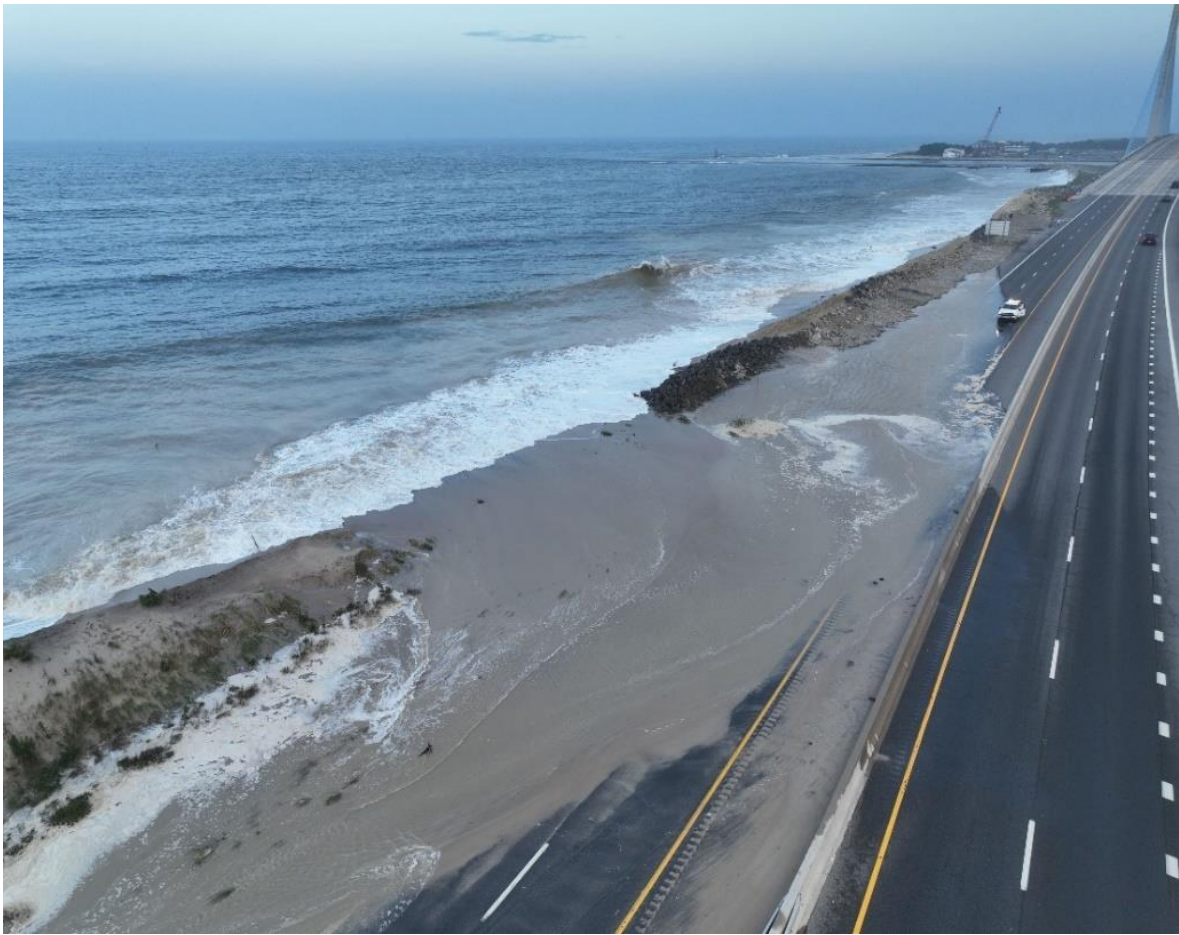
Figure 3. August 17, 2024. View of the dune breach at Delaware Seashore State Park (looking south). The SR-1 northbound lane is covered in water and sand, forcing a road closure.
