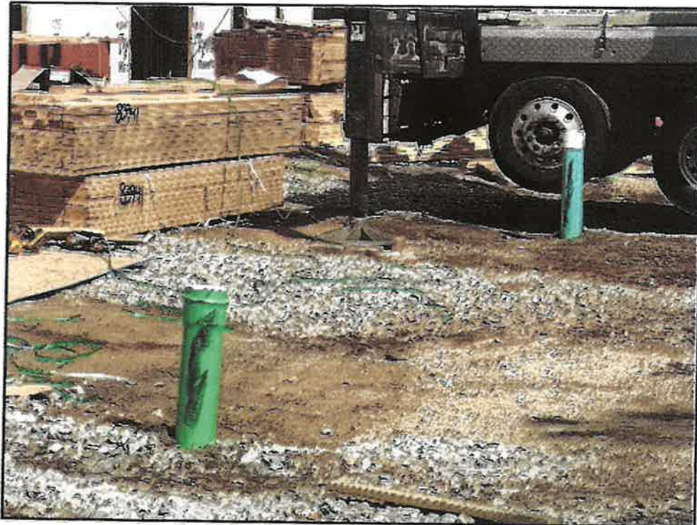
Photograph No. 4 Revised sewer construction in proposed concrete drive and walkway area (439 Bradford Street)
