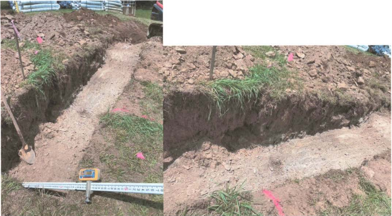
7/10/2023 Trench 1 showing excessive rock.
