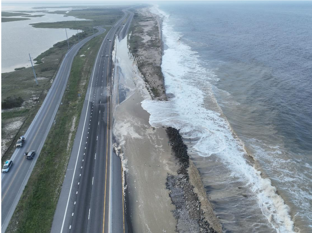
Figure 1. August 17, 2024. Aerial view of the dune breach at Delaware Seashore State Park (looking north). The SR-1 northbound lane is closed to vehicles and completely covered in ocean water, sand, and debris.
