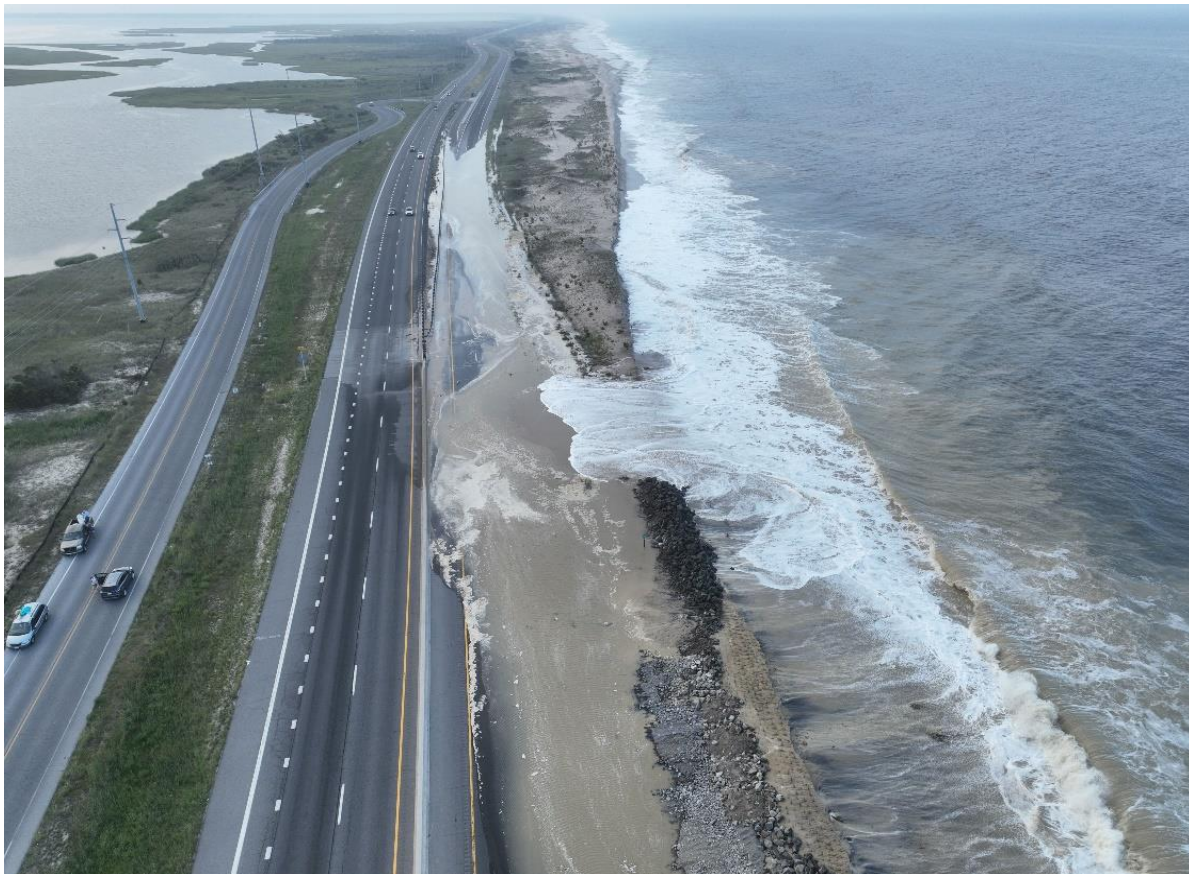
Photo 1. August 17, 2024. Aerial view of the dune breach at Delaware Seashore State Park (looking north). The SR-1 northbound lane is closed to vehicles and completely covered in ocean water, sand, and debris.
