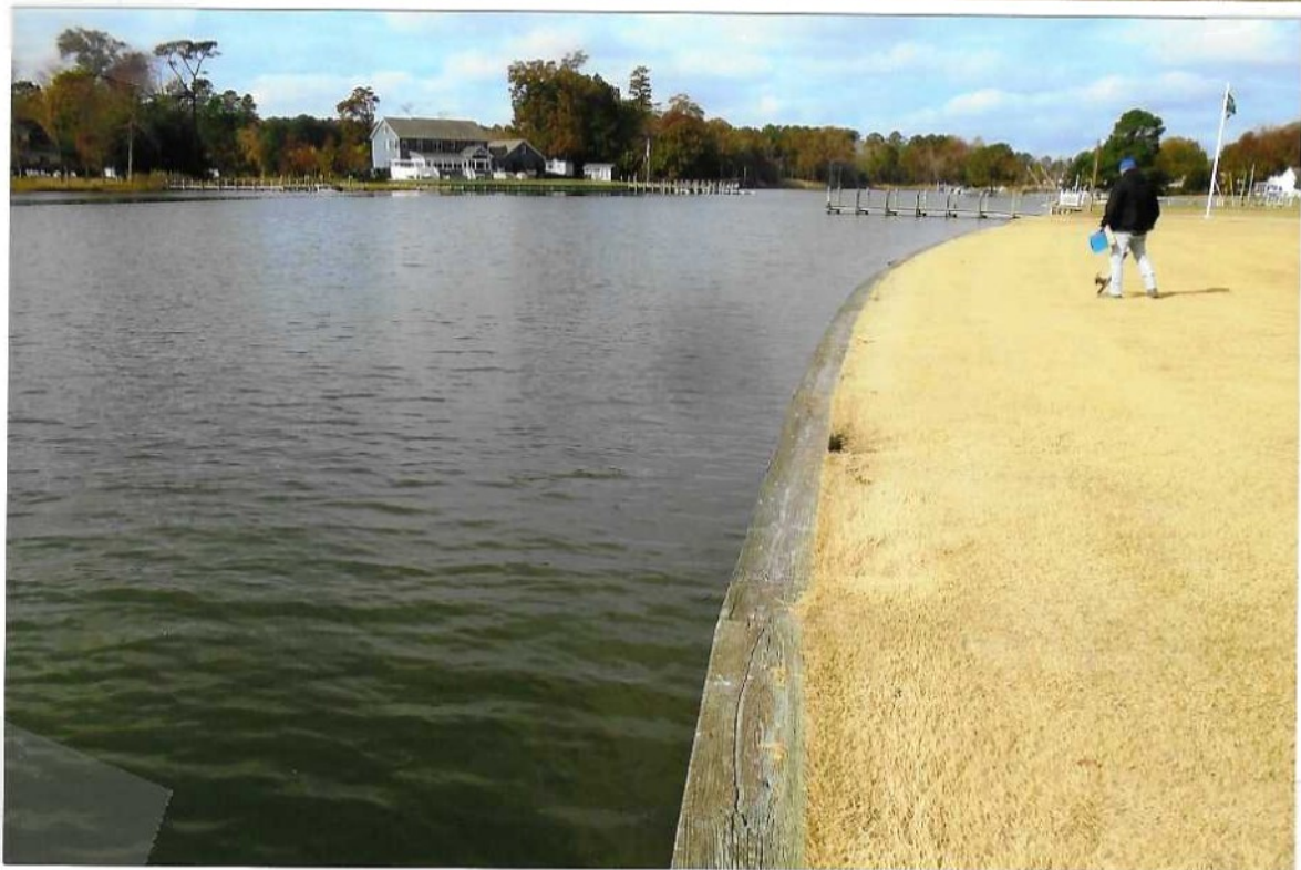
Figure 7. Ground-level photographs of site, 25 Creek Drive, Winding Creek Village, Millsboro, Sussex County, Delaware, adjacent to Guinea Creek. Applicants propose to repair/replace a 188' bulkhead and to construct a 66' long x 4' wide pier; a 6' wide x 24' long dock, and a 4-piling boat lift. See Figure 8 for plan view and cross-section sketches.
