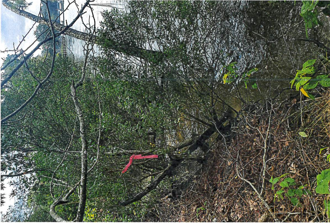
View of eroding vertical bank at high tide.
