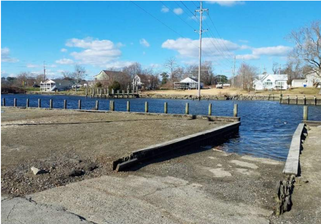
DPL-IR-WC2: Facing northwest showing the E1UBL watercourse and the bulkhead near Pole 72.
