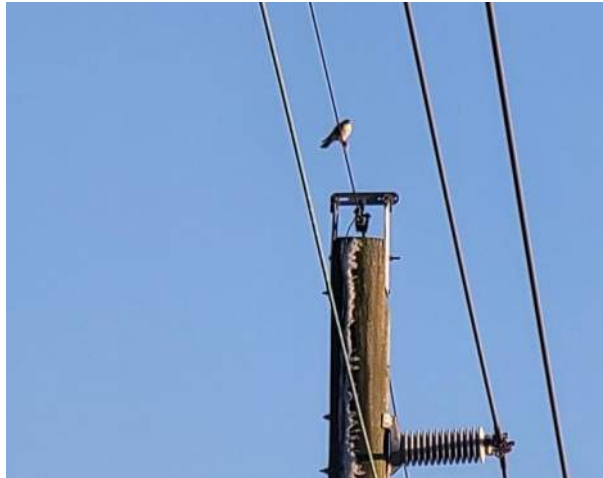
American kestrel perched on a transmission line adjacent to Structure 32.
