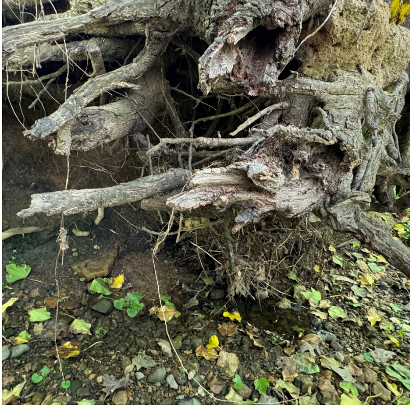
PHOTO 4: EXPOSURE OF TREE ROOTS DUE TO BANK EROSION
