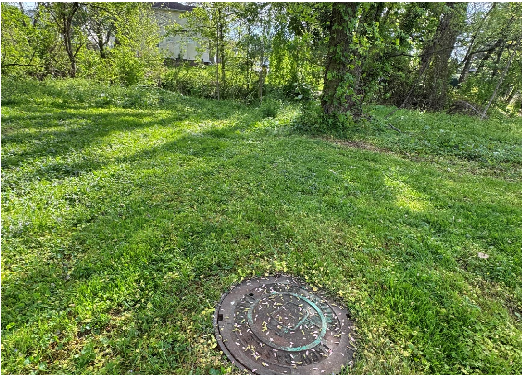
PHOTO 5: SEWER INFRASTRUCTURE IN THE STREAM VALLEY
