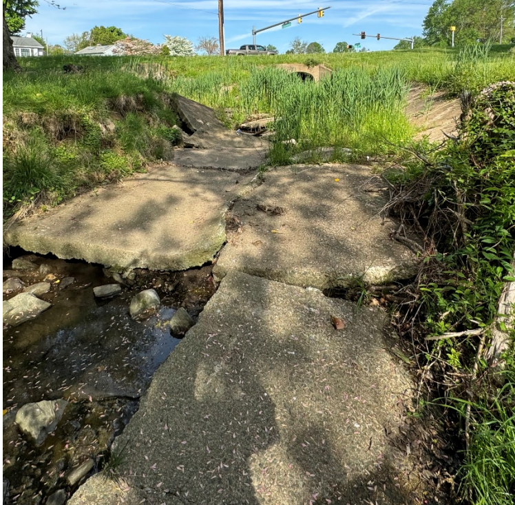
PHOTO 6: FAILED CONCRETE FLUME WITHIN THE EXISTING CHANNEL
