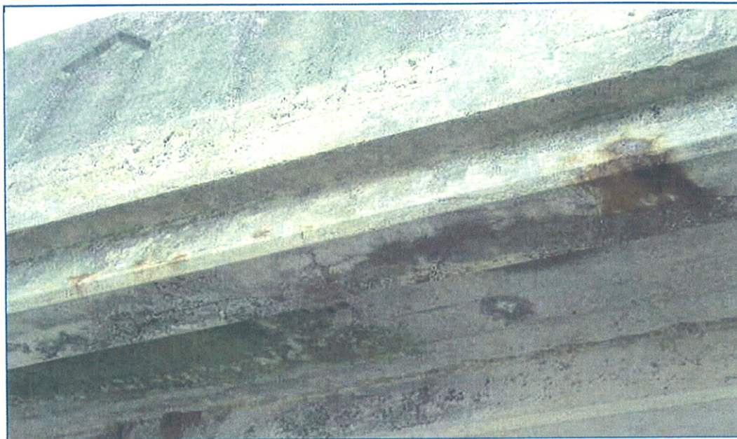
7. CRACKS W/ RUST STAINING IN EAST FASCIA BEAM
