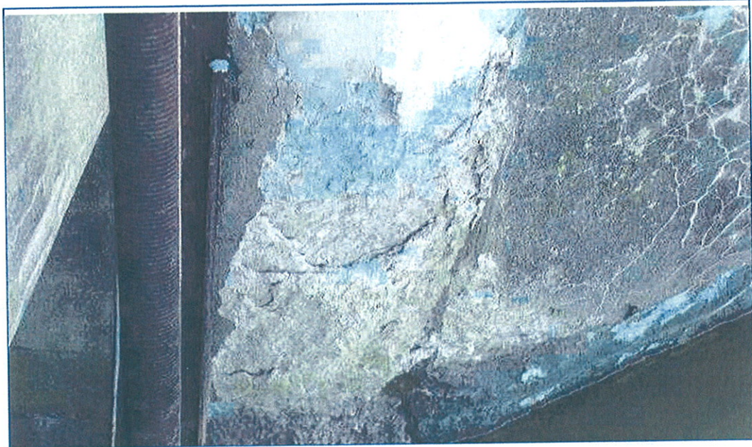
7. DETERIORATED CONCRETE ALONG S/W WINGWALL
