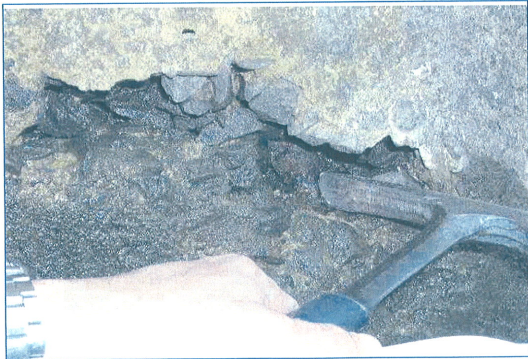
6. DEEP HONEYCOMBING W/ EXPOSED REBAR @ WEST END OF SOUTH CELL
