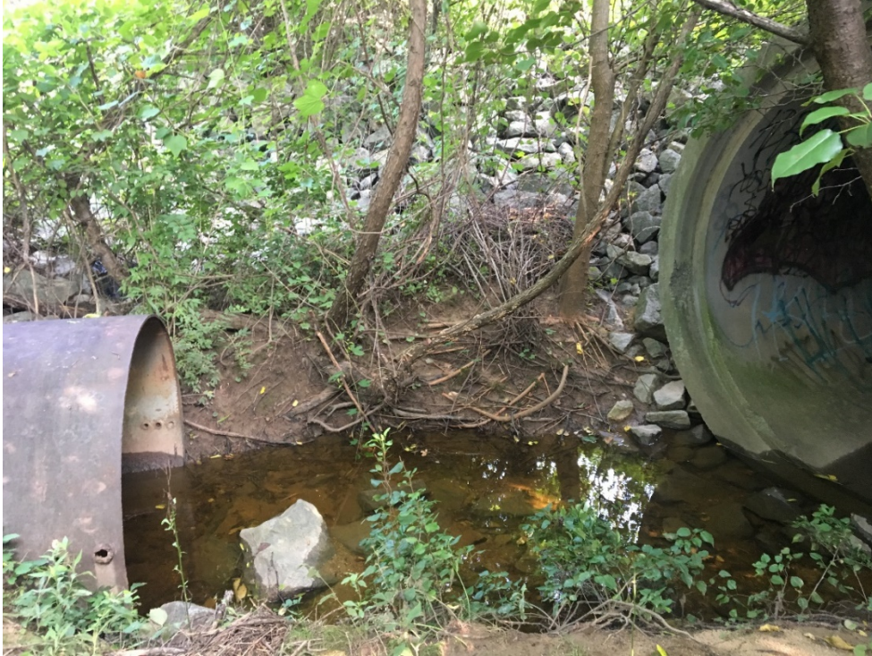
Photograph 4: Flow from the pipe then travels through a second pipe. The second pipe transports flow off the project site, where it eventually drains into Army Creek.
