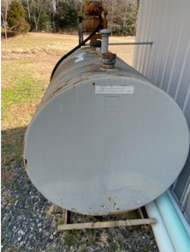
Above ground fuel tank
