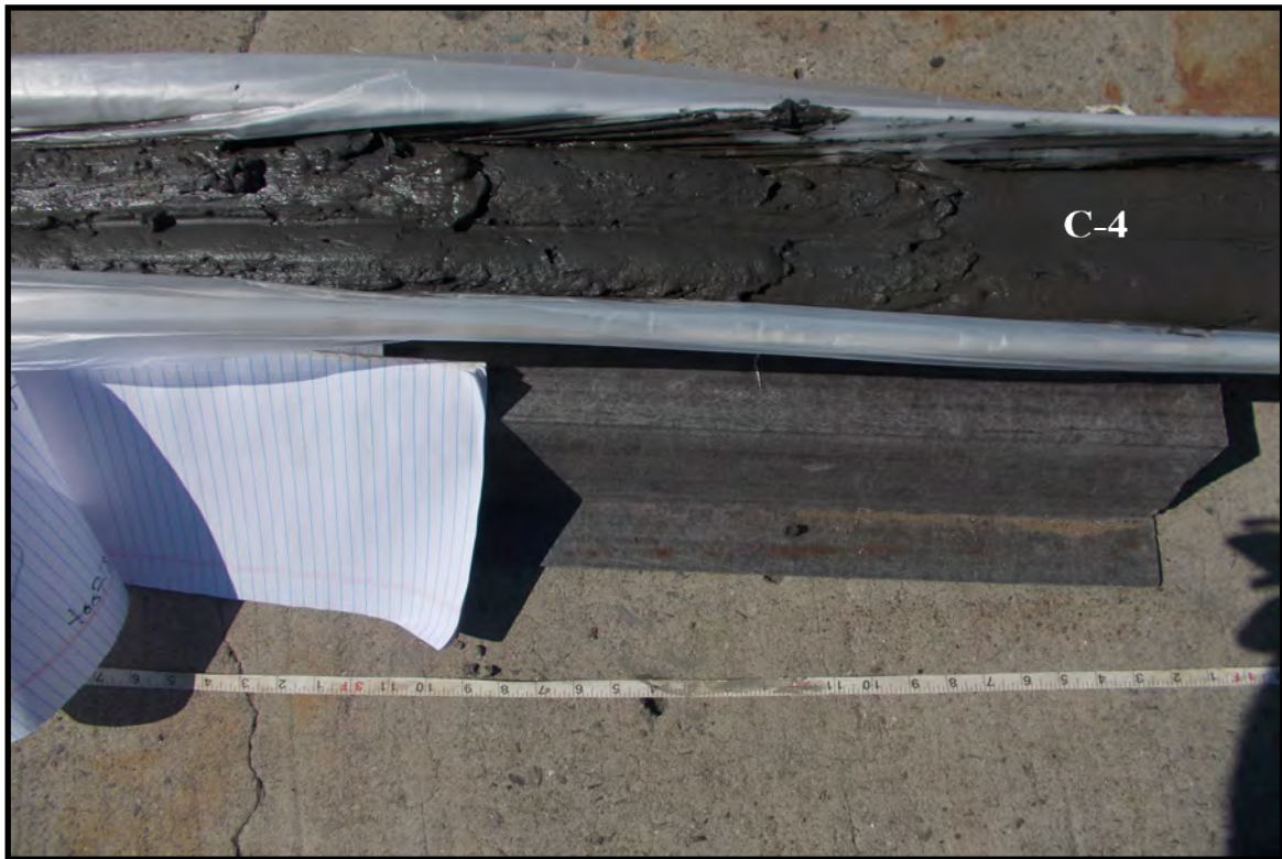
PHOTO No. 16: C-4, CENTER
