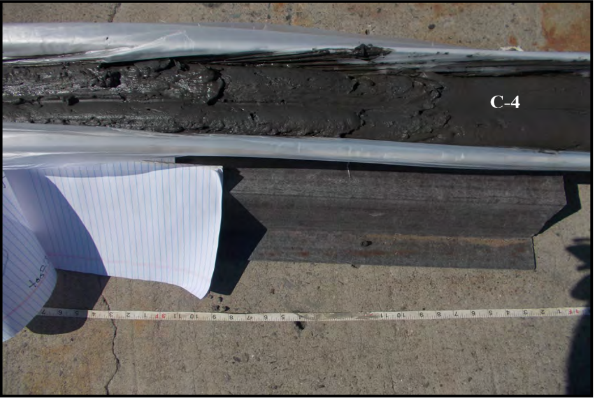
PHOTO No. 16: C-4, CENTER
