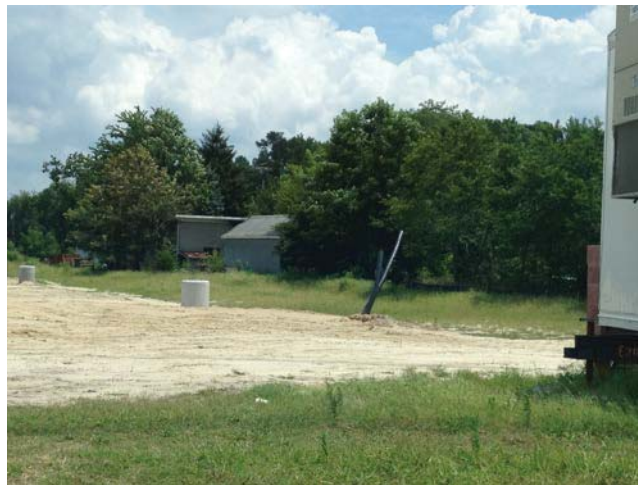
Along Kollock Street where the bare construction area and grass meet with tall trees in the background.
