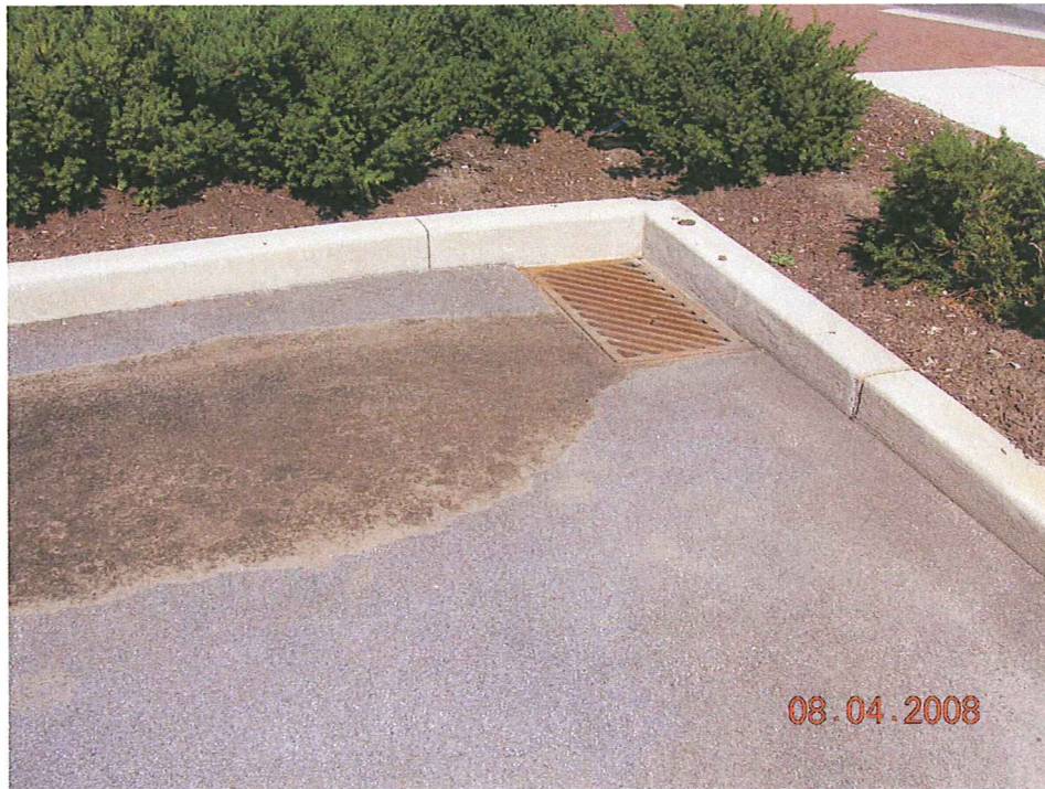
Sediment migrating into drainage basin from ongoing construction activities.
