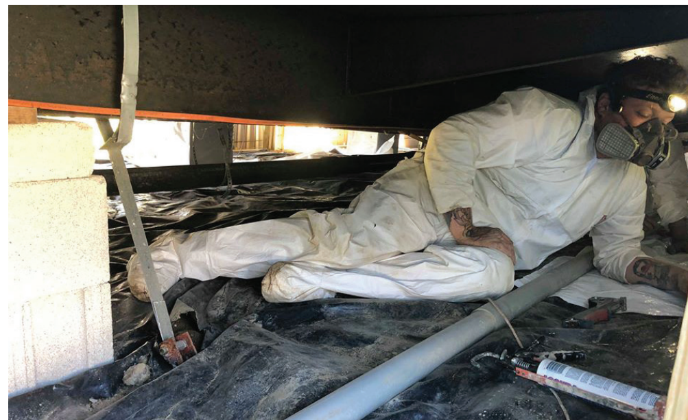
Caulking under a manufactured home.
